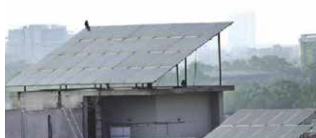
Figure 2: Training Academy Building of BREB's H/Q Rooftop Net Metering Station
