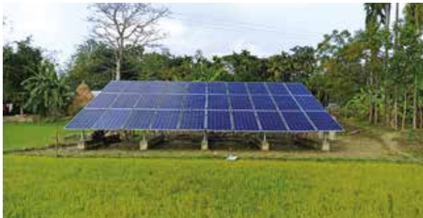
Figure 1: Solar Irrigation Pump at Kishoreganj PBS
