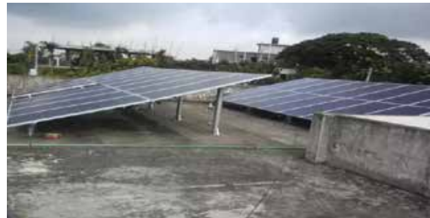
Figure 2: 10 kWp rooftop solar plant with Net metering at Narayanganj PBS-2
