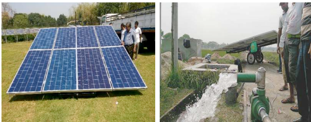
Fig. 60 Portable solar pump irrigation system
